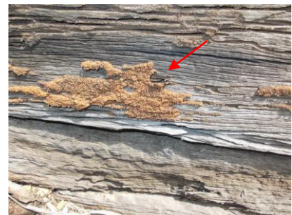
active termites in sleepers
