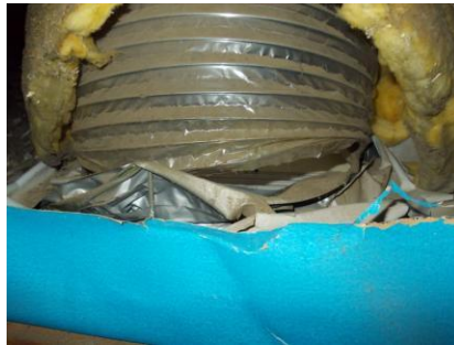
air conditioner duct
