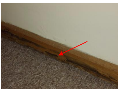
wood decay in skirting board
