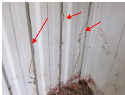
termite mudding on wall of shed
