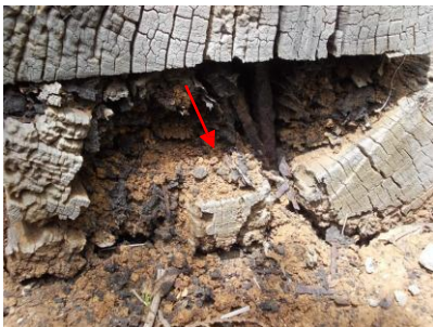
Termite damage to retaining wall
